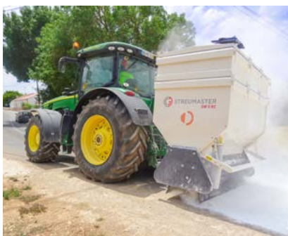
The rear-mounted SW 5 RC binding agent spreader precisely distributes the required amount of lime in front of the cold recycling train. Image source: Wirtgen Group
