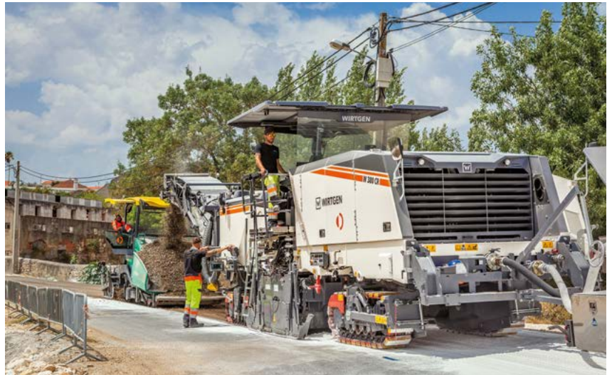
In Monsanto, the powerful Wirtgen W 380 CR with rear loading recycled the pavement to a depth of 16 cm through the addition of foamed bitumen, water and pre-spread lime. Image source: Wirtgen Group
