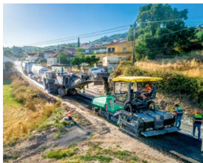
Milling, processing, paving and compacting – eco-friendly road rehabilitation with technology from the Wirtgen Group. Image source: Wirtgen Group
