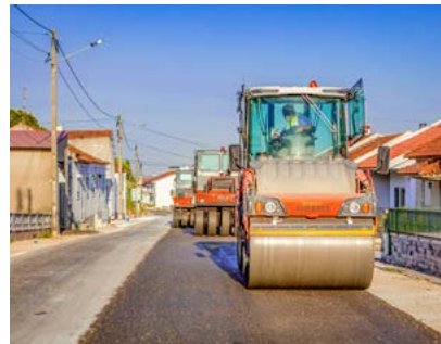
The first compaction passes were carried out with a HD+ 110i tandem roller. Subsequently, two GRW 18 pneumatic tyre rollers were used for final compaction and sealing. Image source: Wirtgen Group
